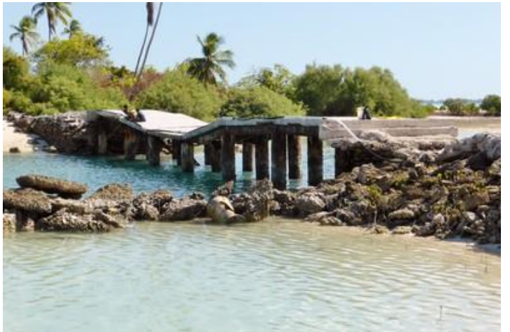
Second pont cassé, North Tarawa, Kiribati
